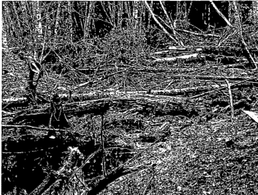
Figure 5.2.30 Log that formed part of the log revetment constructed after the 2006 landslide and found in distal portion of Zone F (note steel cables). Photo taken on May 23, 2014; Camera position: 48.27912°N, 121.83592°W, view toward the northeast.
