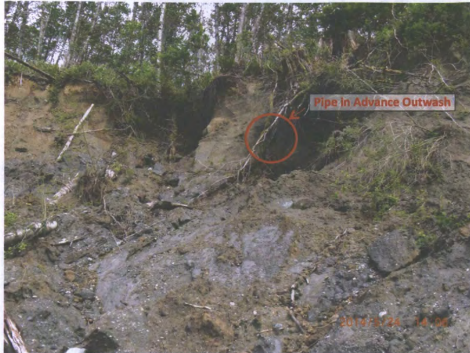
Figure 5.2.14 Seepage and piping near interface between Advance Outwash sand overlying Glacial Lacustrine clay. Location: N 48°17.124' W 121°50.827'; view looking east.
